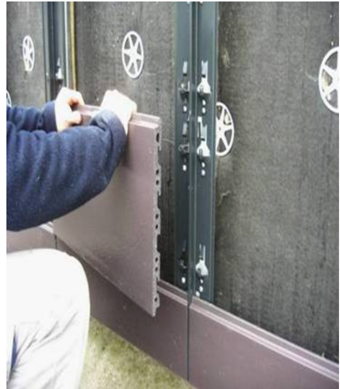
hang on panels
